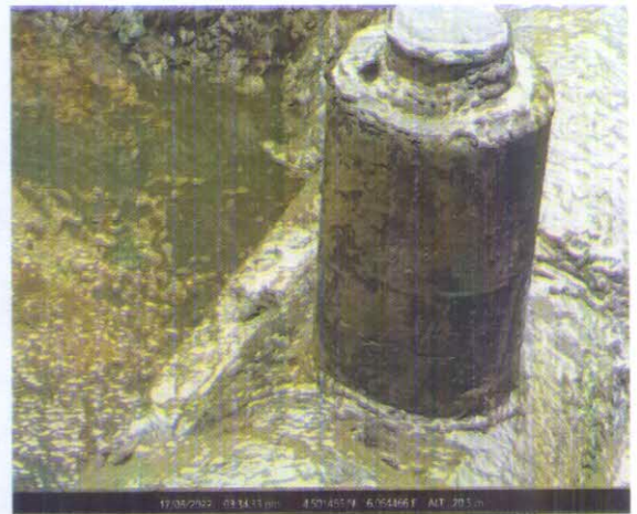
FIG.2 SHOWING SPILL POINT (AFTER EXCAVATION)
